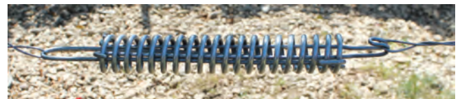
Compensating spring installed on the moveable wire.
